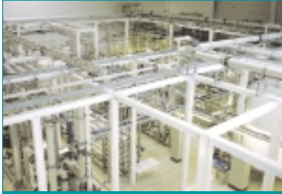
Figure 7. Infineon Technologies Dresden, SC 300: Top View Make-up System.
